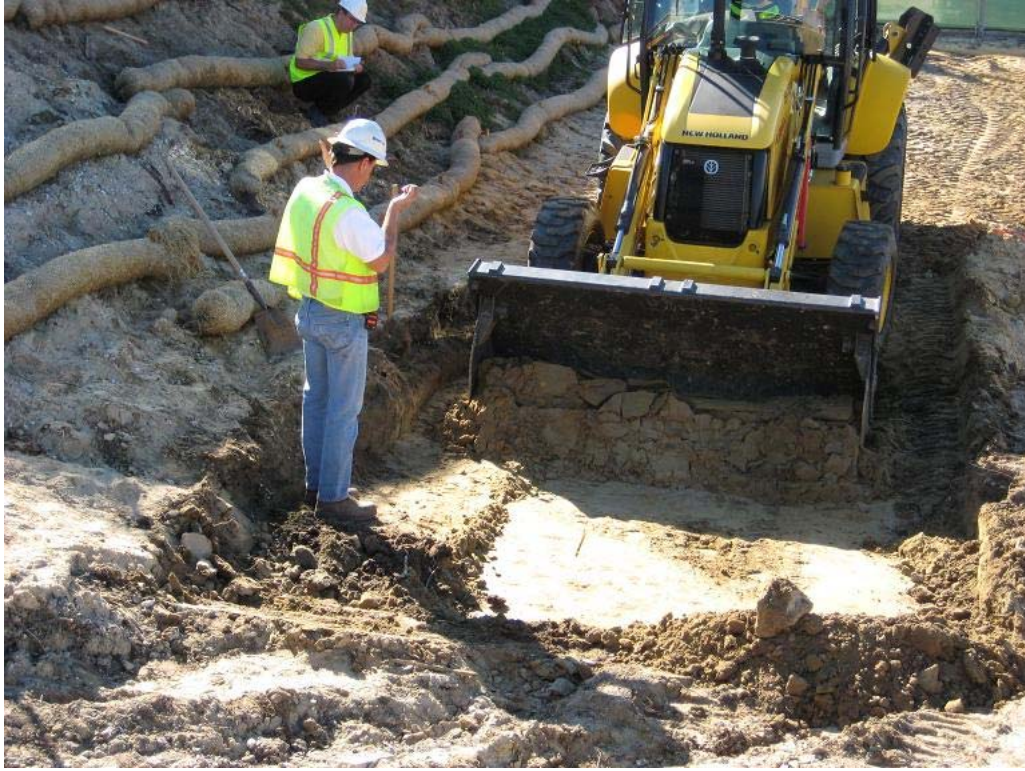
Photograph 1: View to the south of the limited excavation at the northeast corner of 4406 Cather Avenue. Excavation conducted on February 4, 2009.
