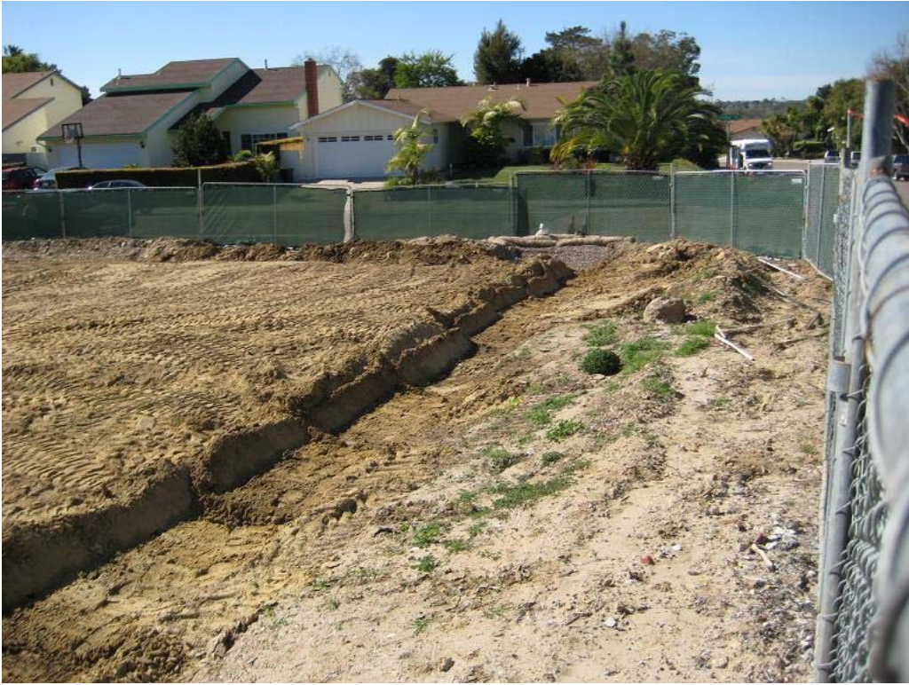
Photograph 7: View to the west toward Cather Avenue of the temporary storm water diversion channel along the northern extent of 4406 Cather Avenue.
