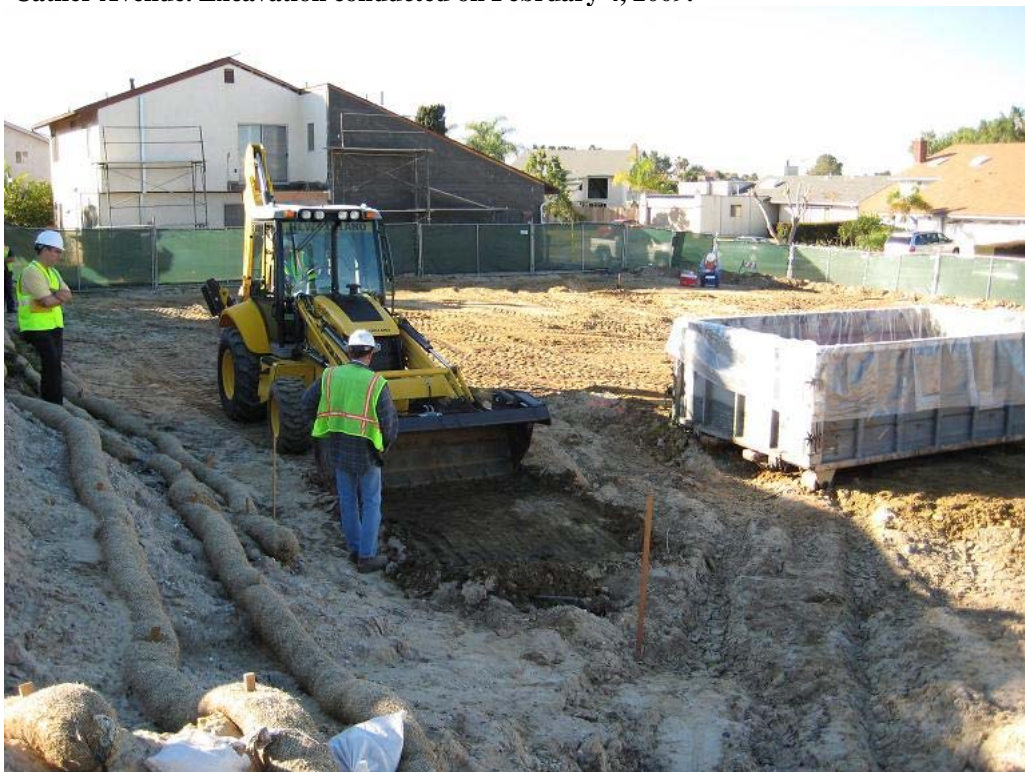
Photograph 2: View to the southwest of the limited excavation at the northeast corner of 4406 Cather Avenue.
